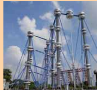
HVDC Generator at UHVRL, Hyderabad
