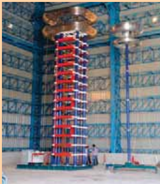
2400kV, 240kJ Impulse Voltage Generator
