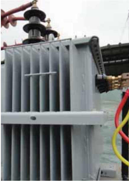
Transformer installed outdoor...
