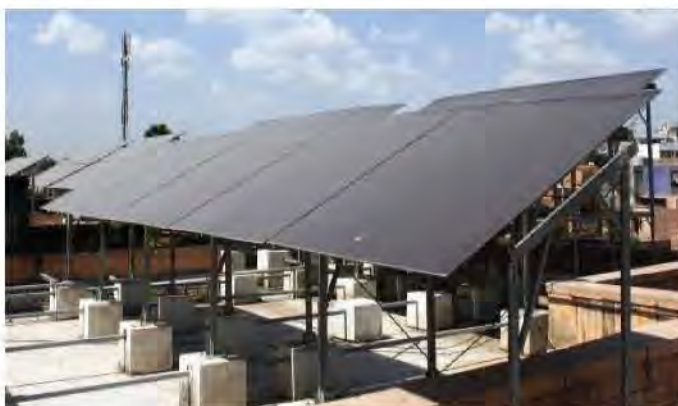
Fig. 5: A-Si based 43 kW rooftop grid tied solar photo voltaic system
