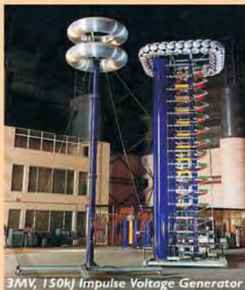
3MV, 150kJ Impulse Voltage Generator
