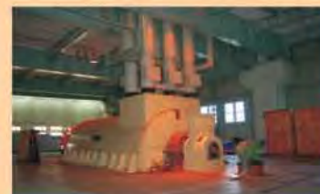
2500MVA Short Circuit Generator
