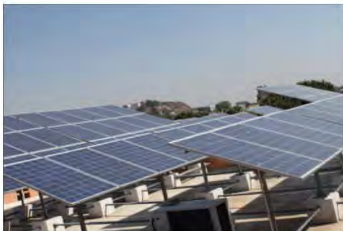
Fig. 2: C-Si based 58 kW rooftop grid tied solar photo voltaic plant
