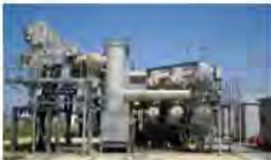
420kV, 63kA Gas Insulated Switchgear
