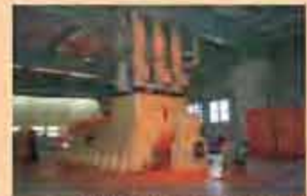
250MVA Short Circuit Generator
