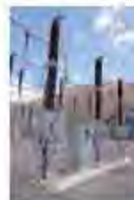
215kV Live Tank Circuit Breakers
