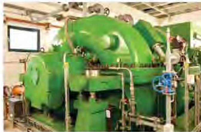
Fig. 2: Top Pressure Recovery Turbine
