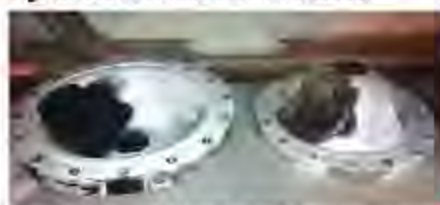
Fig. 1: Surface carbon deposition due to failure arcs
