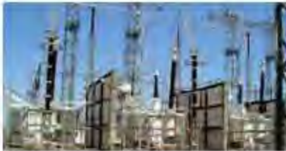
1650MVA, 765kV Class Power Transformers
