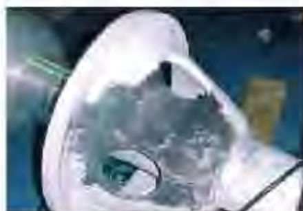
Fig. 1: Traces of flashover on a busbar
