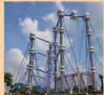
HVDC Generator at UHVRL, Hyderabad
