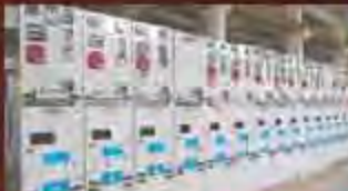
Sudhir-Schneider HT Panels
