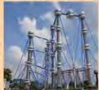
HVDC Generator at UHVRL, Hyderabad
