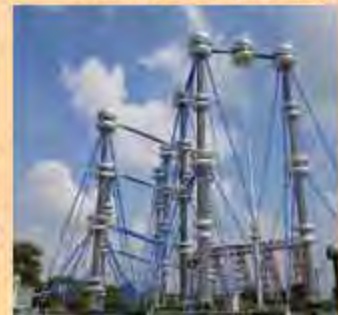
HVDC Generator at LHVRL, Hyderabad
