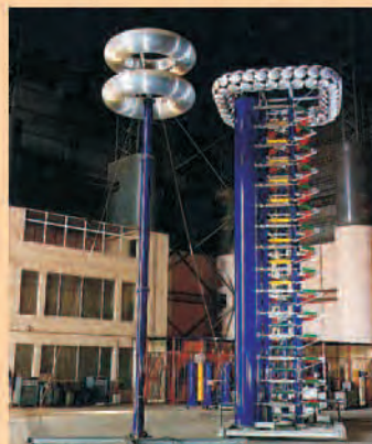
3MV, 150kJ Impulse Voltage Generator
