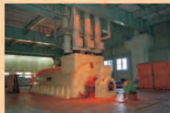
2500MVA Short Circuit Generator
