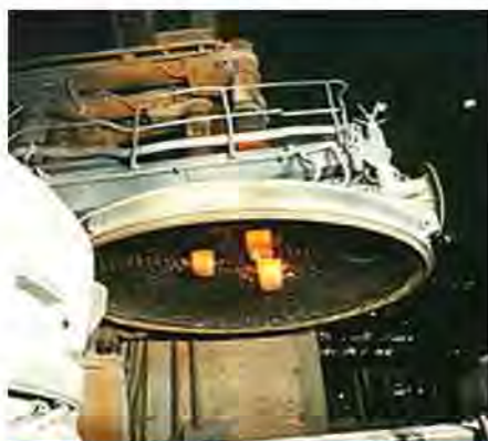
Fig. 3: Water cooled swung out roof of an EAF, showing the three electrodes.
