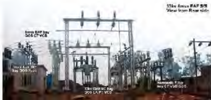
Fig. 8: 6mva, 33kv EAF substation with Harmonic Filter (view from front)
