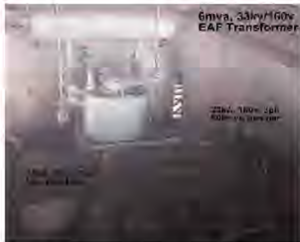
Fig. 5: EAF Transformer, 3ph, 6mva, 50Hz, 33kv/160V
