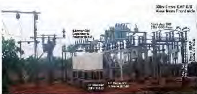
Fig. 9: 6mva, 33kv EAF substation with Harmonic Filter (view from rear)
