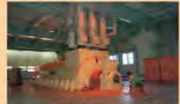
2500MVA Short Circuit Generator
