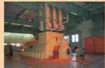
2500MVA Short Circuit Generator
