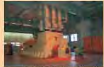
2500MVA Short Circuit Generator
