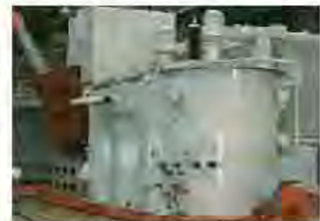
Toshiba 15/150 MVA 110 KV GIT in underground substation)... (Low pressure Design 0.14 MPa-g)
