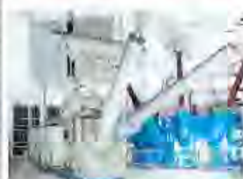
World's first successfully tested converter and transformers connecting 800 kV UHVDC with 750 kV AC...
