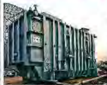
Alstom's HVDC power transformer for the Champa project...
