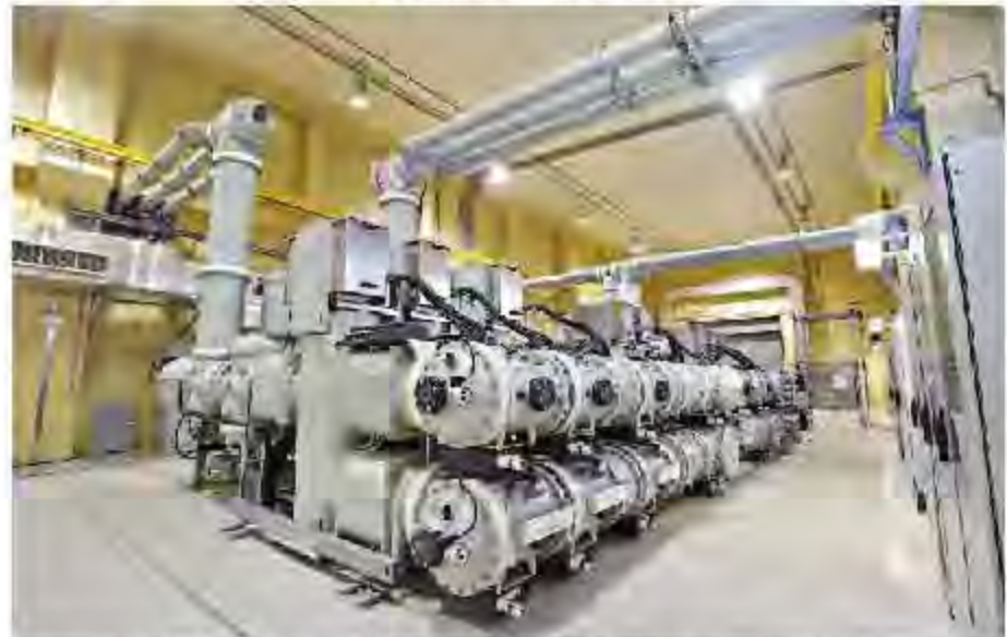
Alstom Gas Insulated Transformers at 145kV Gas-insulated switchgear (F35) at the Shuqaiq HV substation in Saudi Arabia...
