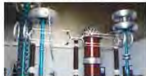
400kV Transmission Line Hardware under HV Test
