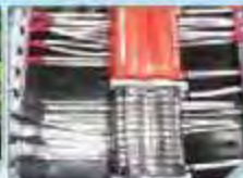
Control panel near generation terminals
