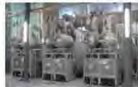
Toshiba 400 MVA GIT in underground substation)... (High Pressure Design 0.43 MPa-g)
