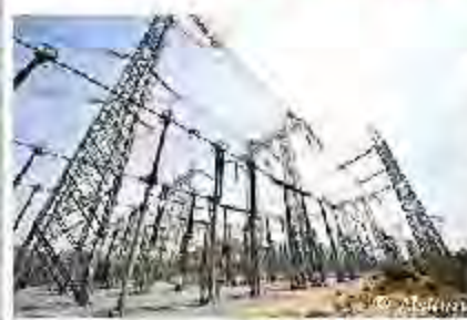
Overview of an AIS substation...
