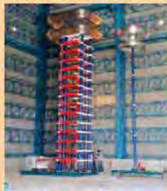
240kV, 240kJ Impulse Voltage Generator
