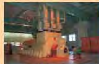
2500MVA Short Circuit Generator
