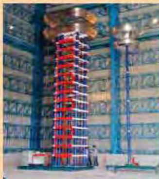
2400kV, 240kJ Impulse Voltage Generator
