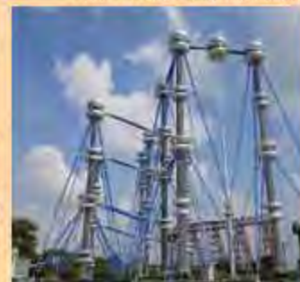
HVDC Generator at UHVRL, Hyderabad
