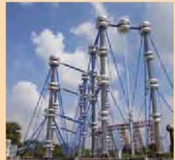
HVDC Generator at UHVRL, Hyderabad
