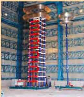
2400kV, 240kJ Impulse Voltage Generator
