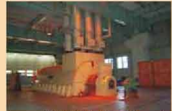
2500MVA Short Circuit Generator
