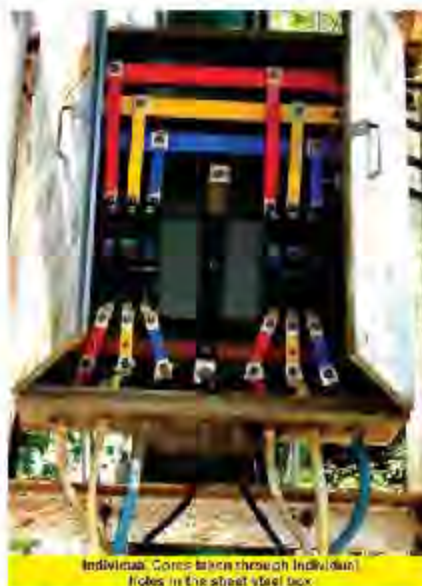
Fig. 5: Pole Mounted Sheet steel box showing Transformer Secondary side circuit breakers feeding two separate feeders
