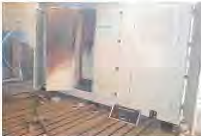
Photograph of Package substation after test
