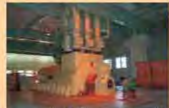
2500kVA Short Circuit Generator
