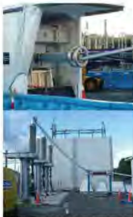
Fig. 1: Resonance test set connected to the cable termination current transformers (HFCTs) to pick up the PD signal with high efficiency (See Figure 2).
