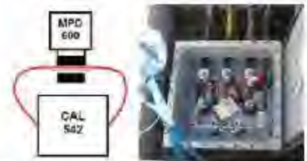
Fig. 3: Performance checks of HFCT sensors
