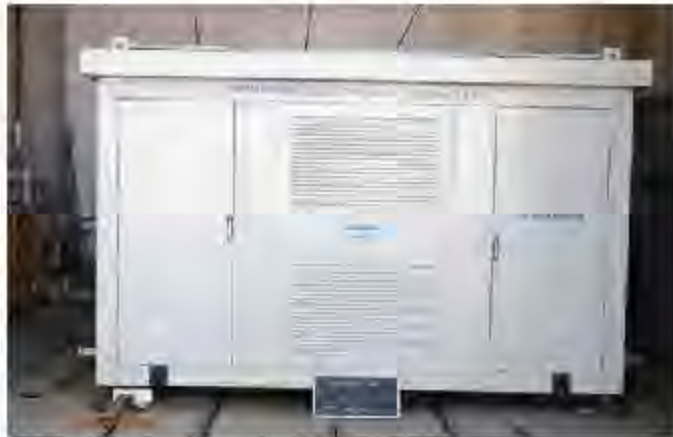
Photograph of Package substation before test
