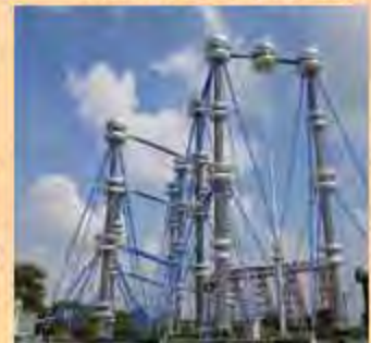
HVDC Generator at LHVRL, Hyderabad
