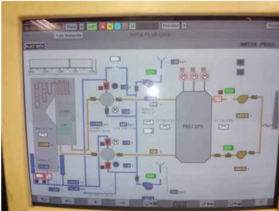
Figure 5: View of console a typical control panel in a coal power plant...
