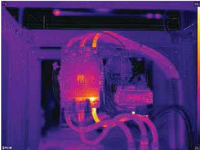
Contactor with pronounced abnormality of the right phase on the lower terminal connection. The possible cause could be increased resistance at the terminal connection, an internal connection or the contactor. The labels are also easily recognizable here thanks to the MSX feature...
