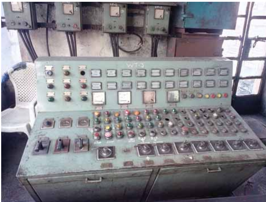
Figure 6: Older design of control panel of a coal handling plant in a power station...
