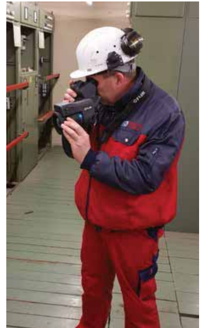
Martin Adler taking thermal images of a low-voltage main distribution...
