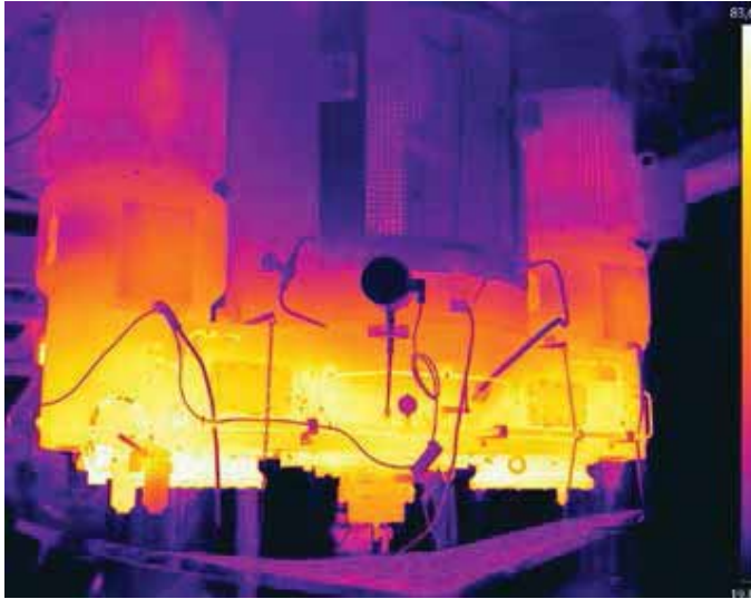
Agitator drives below a mixing tank in an area at risk of explosion in a chemical operation...
