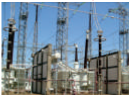
1650MVA, 765kV Class Power Transformers
