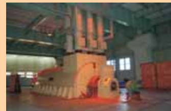
2500MVA Short Circuit Generator
