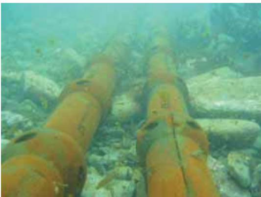
Armoured sub sea cables at EMEC...
