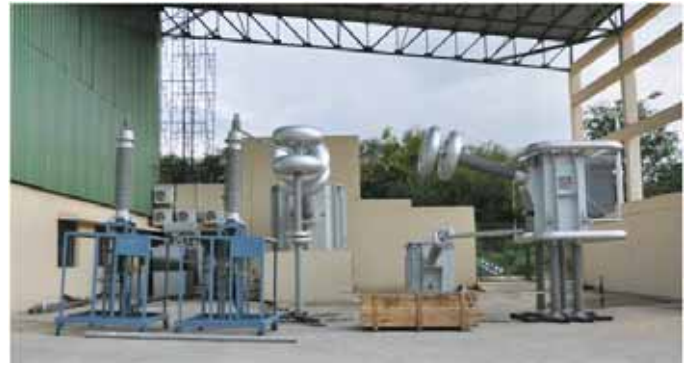
Figure 8. Outdoor 600 kV, 4200 KVA transformer for conducting pre-qualification test...
