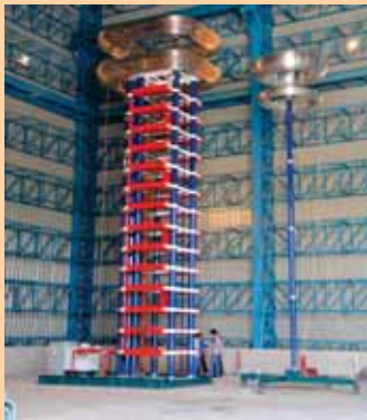
2400kV, 240kJ Impulse Voltage Generator
