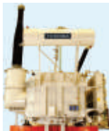
333MVA, 1200kV Single Phase Auto Transformers
