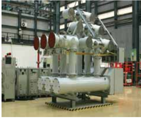
Gas Insulated Switchgears
