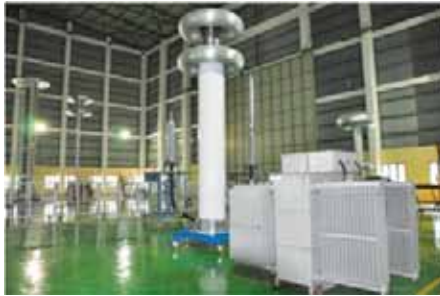
Figure 7: A view of high voltage indoor lab 2400 kV, 240 kJ..
