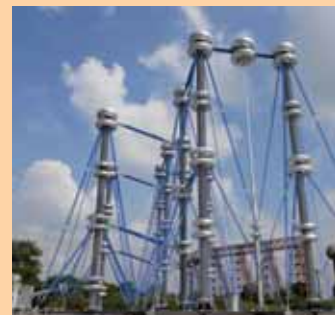
HVDC Generator at UHVRL, Hyderabad
