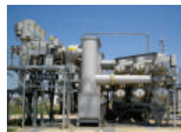
420kV, 63kA Gas Insulated Switchgear
