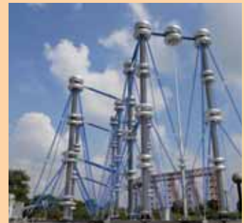
HVDC Generator at UHVRL, Hyderabad
