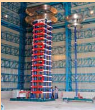
2400kV, 240kJ Impulse Voltage Generator
