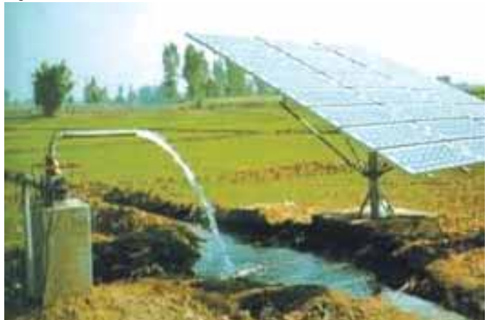
Figure 5 Water pumping with solar system...
