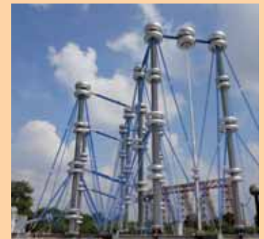
HVDC Generator at UHVRL, Hyderabad
