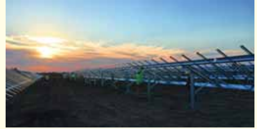
Solar FlexRack Installed in the largest solar project in Iowa
