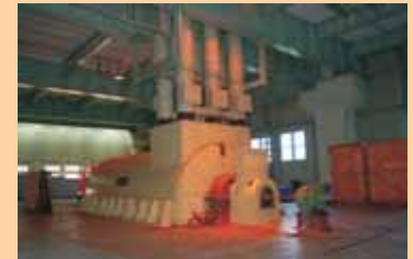
2500MVA Short Circuit Generator
