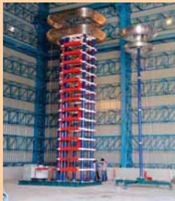
2400kV, 240kJ Impulse Voltage Generator
