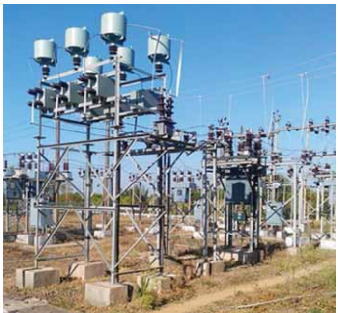
Figure 1: Typical Capacitor Bank Installation
