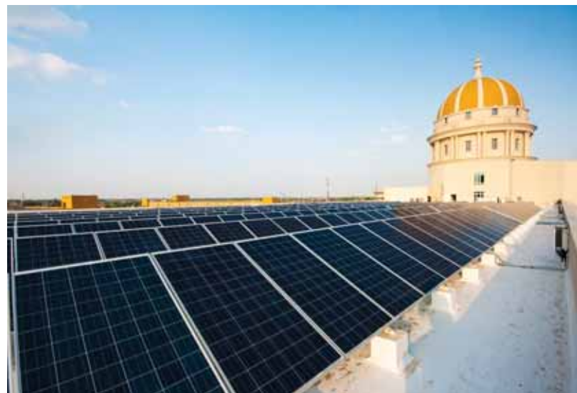
Manipal University Jaipur - 800 kWp
