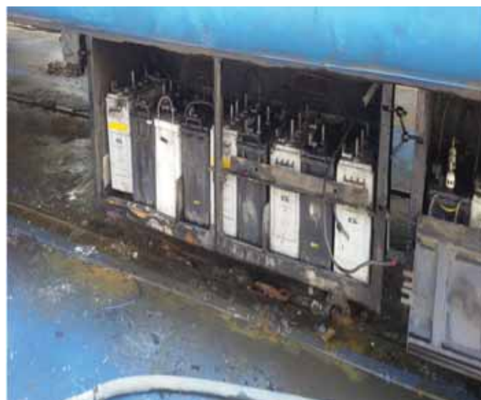
Fig 2: Location of batteries in railway coaches...
