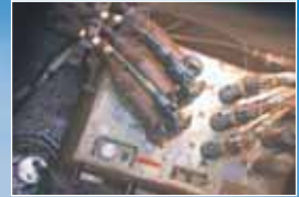
Substation three phase recloser
