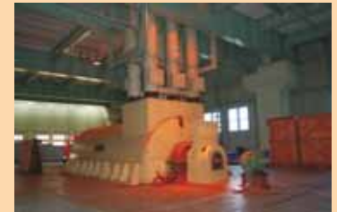
2500MVA Short Circuit Generator
