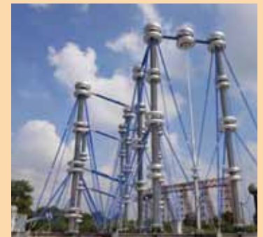
HVDC Generator at UHVRL, Hyderabad
