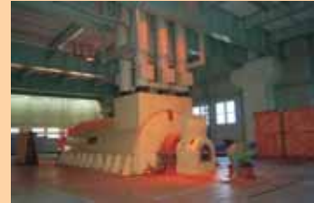
2500MVA Short Circuit Generator
