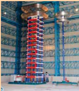
2400kV, 240kJ Impulse Voltage Generator
