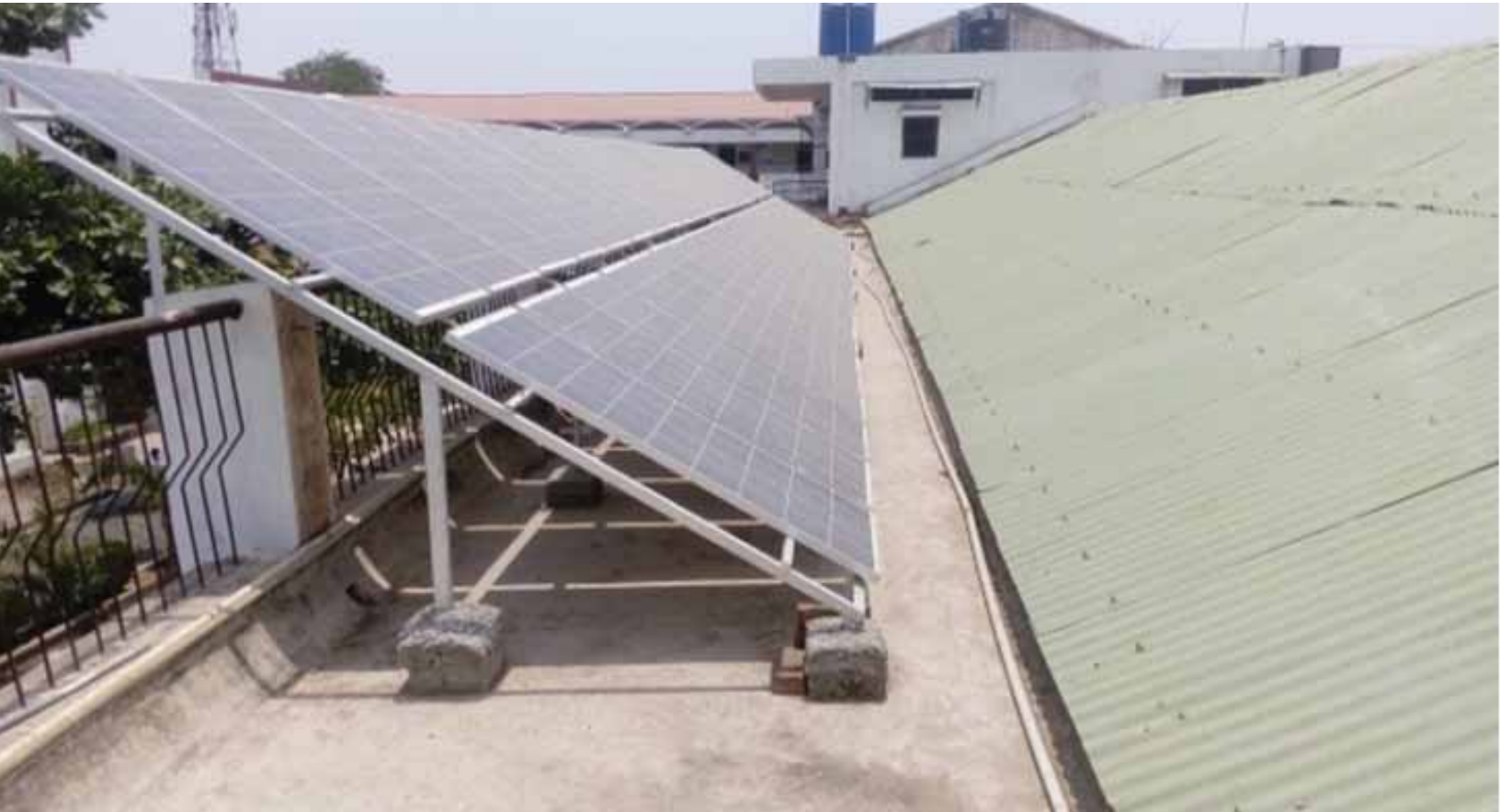
Erected Solar Panels on Terrace of Shri Shivaji College, Akola...
