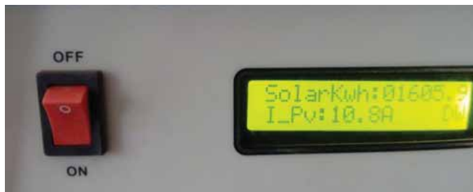
Fig. 4: LCD Display for Solar System Readings...
