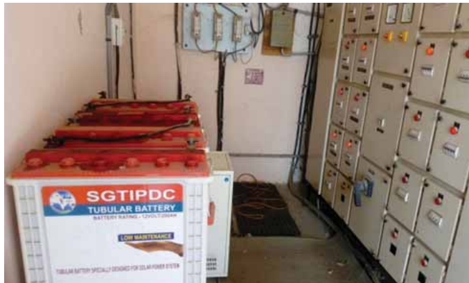
Fig. 3: PCU with Battery in Control Room...
