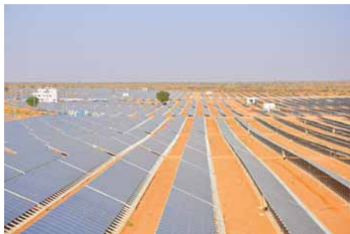
Rajasthan Solar Project
