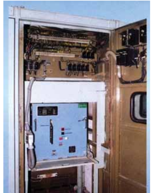
Figure 4: Cassette Mounted VCB
