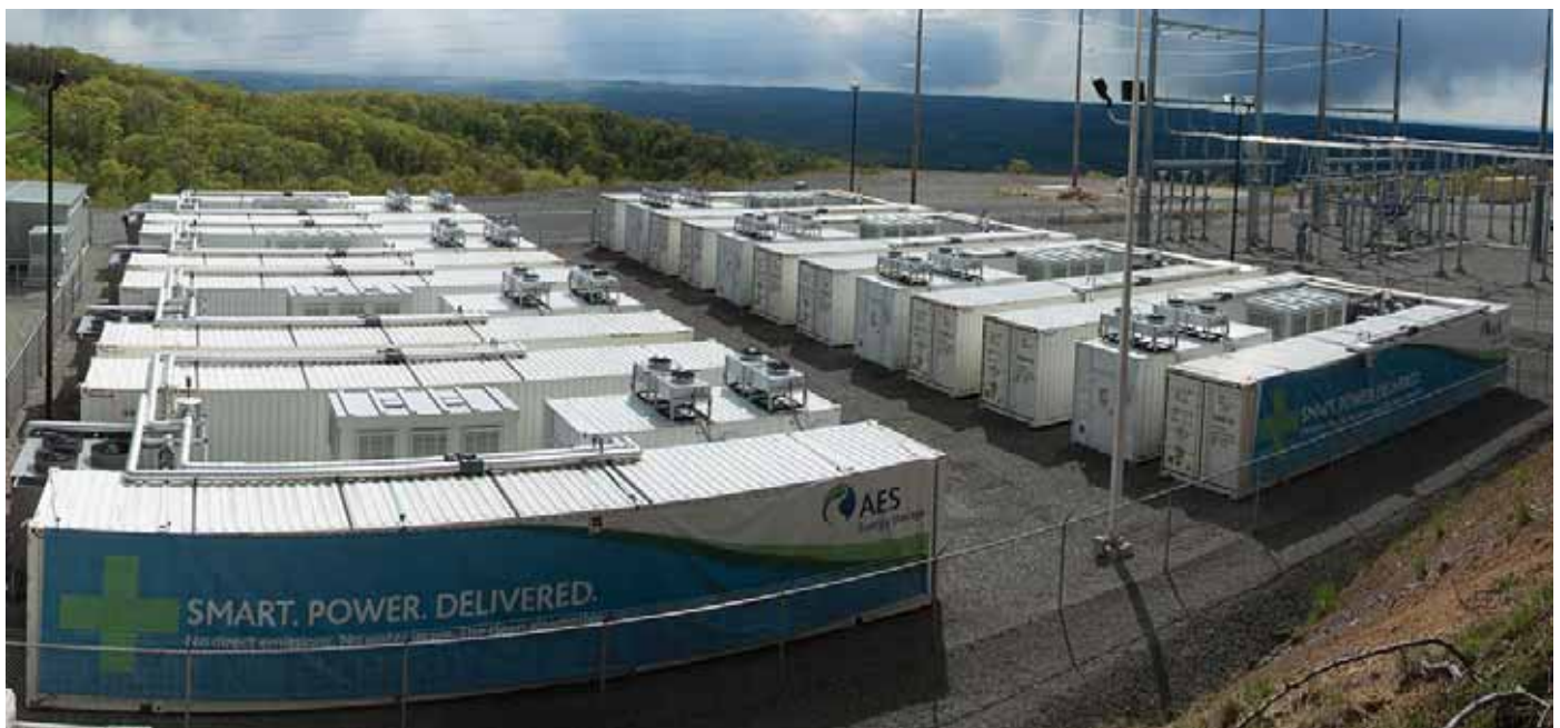
Figure 2: 32 MW 8 MWH Li-ion Battery System by AES at Laurel Mountain, W. Virginia, as energy storage for 110 MW wind farm to maintain frequency. (Source: AES)
