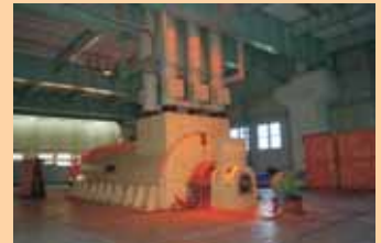
2500MVA Short Circuit Generator
