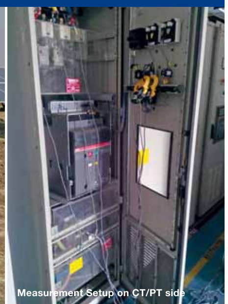
Power Quality Measurement Team with Customer at Solar PV Site
