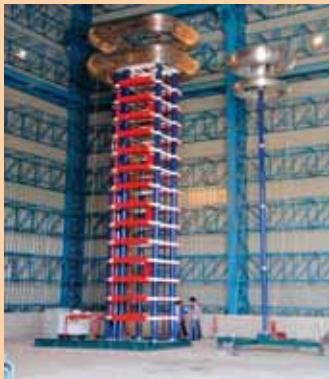
2400kV, 240kJ Impulse Voltage Generator
