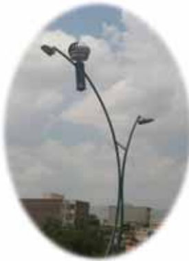
Figure 20: Street Light Luminaires
