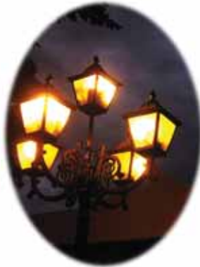
Figure 19: Yard Light Luminaires
