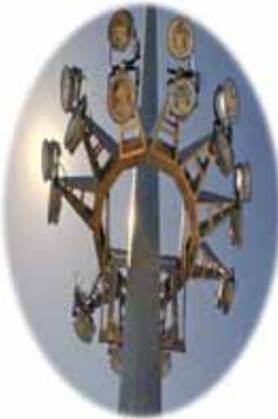
Figure 18: High Mast Luminaires
