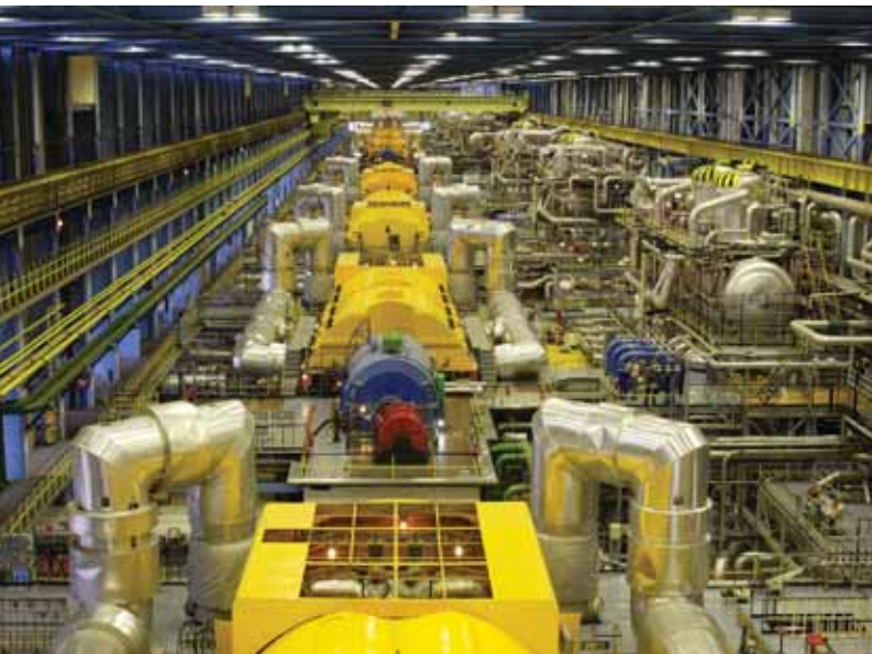
Paks Nuclear Power Plant - Nuclear Hall
