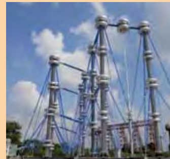
HVDC Generator at UHVRL, Hyderabad
