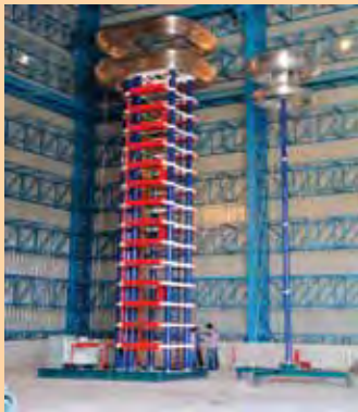
2400kV, 240kJ Impulse Voltage Generator
