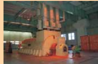
2500MVA Short Circuit Generator
